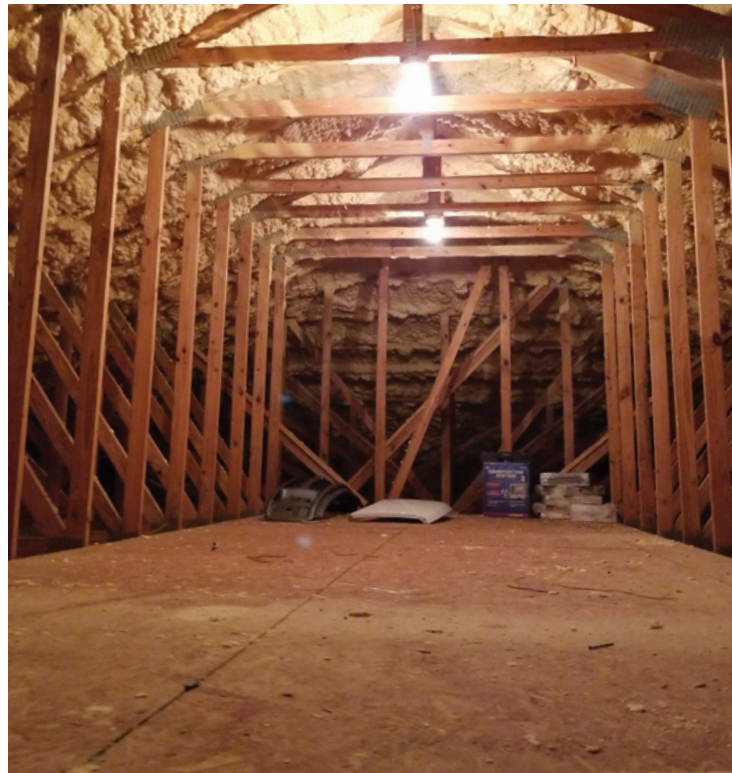
Berry opted to beef up the attic joists so the ceiling structure could handle the tremendous torque that the six enormous fan blades of the Big Ass Fan produce.
