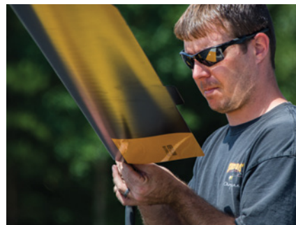
A damaged, worn or improperly balanced rotor will create excessive vibration levels, which can fatigue the flight crew and shorten the service life of the rotor and other parts of the assembly. ACES Image.
