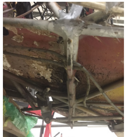
Corrosion and age.
