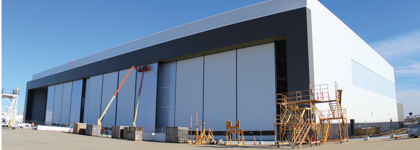
Shown above is Haeco Aero's new Hangar 4, their fifth hangar in Greensboro, currently under construction. It will serve the same role as their existing hangars, which is heavy airframe maintenance. (HAECO Aero image)
