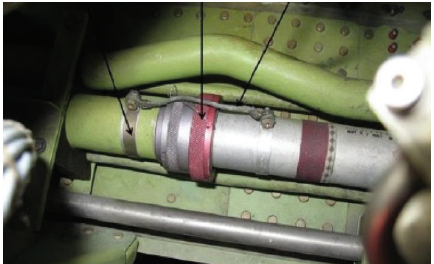
Graphic 6. Exemplar fuel of the coupling and bonding jumper from the RIGHT engine. Note that the lockwire and bonding jumper are properly installed.
