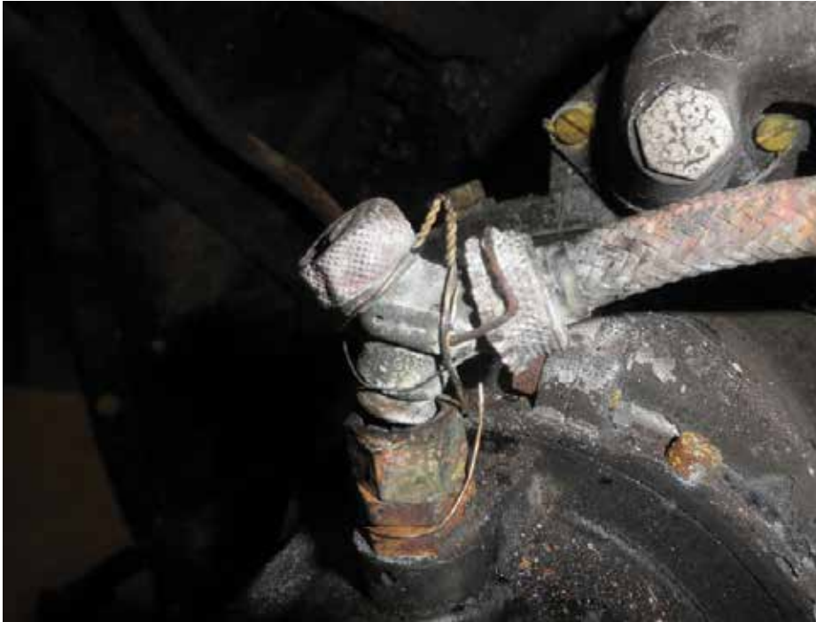
Photo 10: Close-up of the No. 4 engine's left magneto, showing P-lead pulled out of the fitting and with a single strand of safety wire wrapped around the head.
