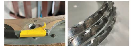
Challenger 300/350 Engine Mounting Ring Corrosion
